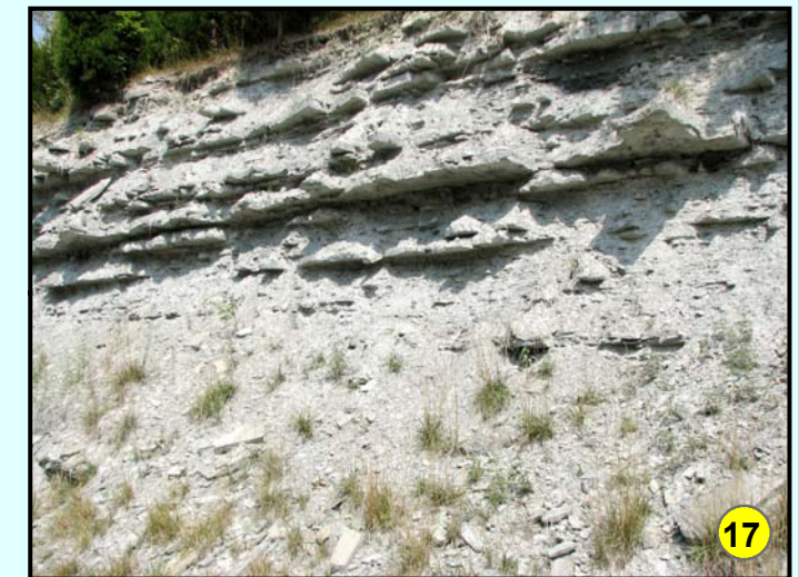
Mile 39.0: Clays Ferry Formation (Ocf); interbedded limestone and shale. Shale beds between the limestone are thicker in the Clays Ferry. When exposed to air and water, the shale breaks down quickly, which leaves overlying limestone layers with no support, and they collapse. This process creates a more rugged terrain, and the rolling Outer Bluegrass is transformed into the Bluegrass Hills (Eden Shale Belt).
