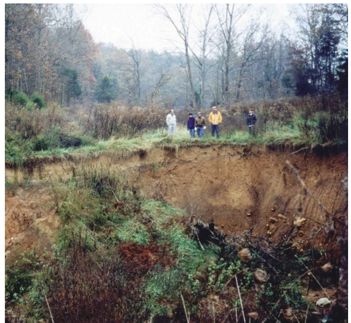
Cover-collapse sinkholes form when the ground caves in, exposing openings in the limestone below. These openings can expand over time, making sinkholes a continuing hazard in karst terrain.
