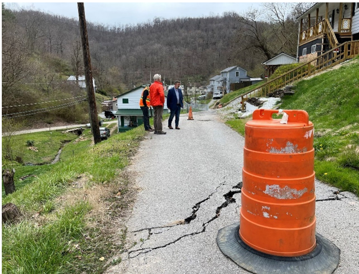
Figure 2. Home and roadway impacted by a landslide (rotational slump) in Jenkins, Letcher County. Photo by Matt Crawford.
