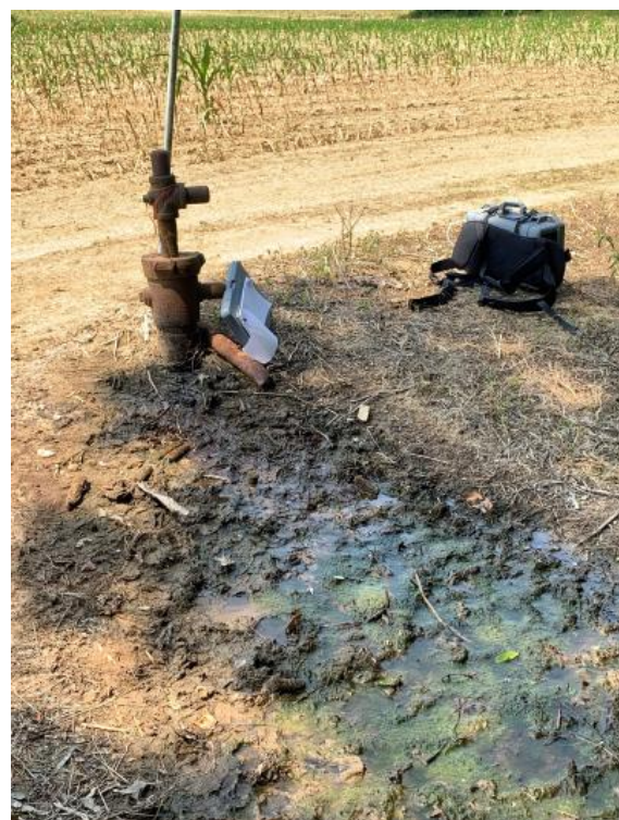
Figure 13. Permit #15297 in McLean County with brine leaking from base of well.
