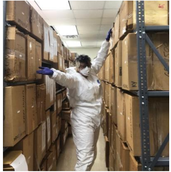
Figure 51. Cheyenne clearing out moldy material damaged during a water leak in the ceiling.
