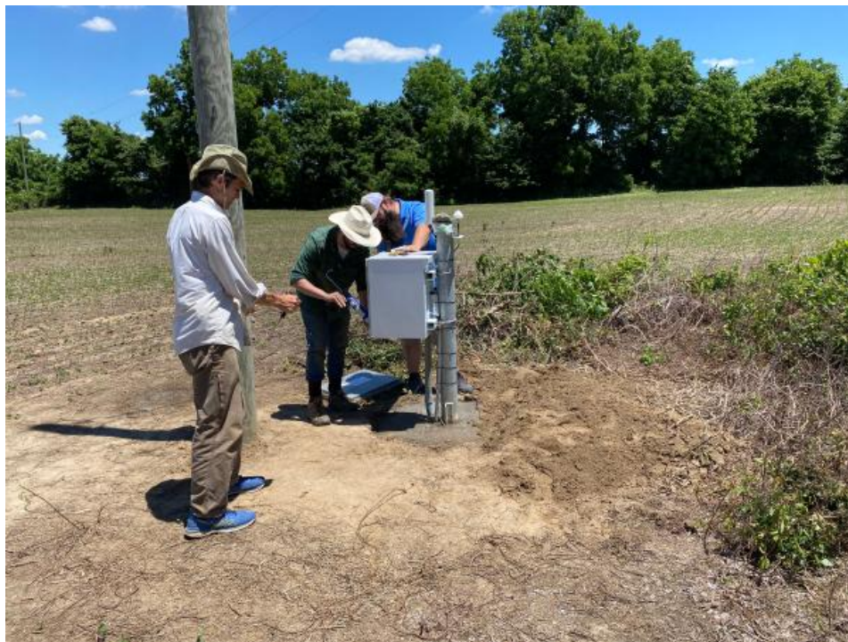
Seth Carpenter, Jon Schmidt, and Russel Rogers installing the strong-motion station, KBKY, in the Kentucky Bend of the most western part of Kentucky and the center of New Madrid Seismic Zone (photo by Zhenming Wang)
