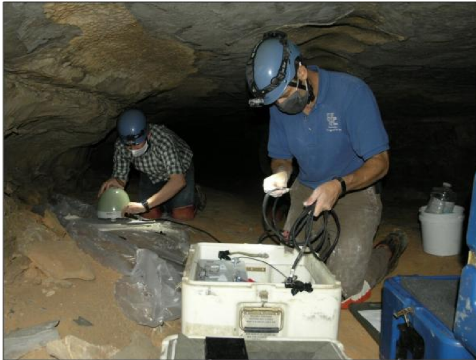
Seth Carpenter (right) and Jon Schmidt install a temporary seismic station in Miller Avenue of Mammoth Cave National Park. Photo by Zhenming Wang .
