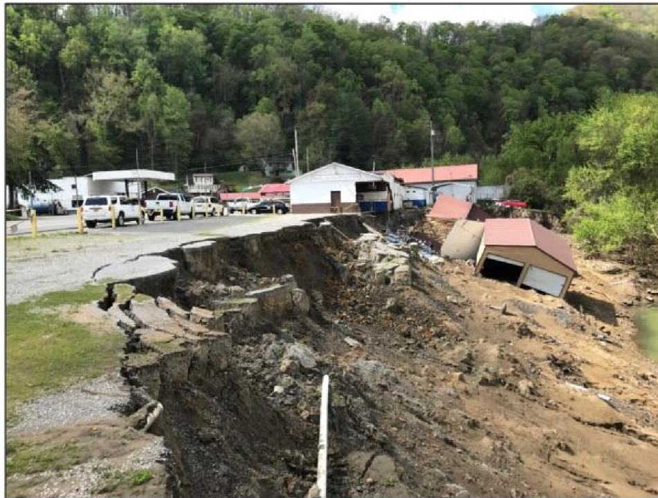
A landslide/river bank collapse in Pike County, Kentucky, in April 2021. Photo by Matt Crawford .
