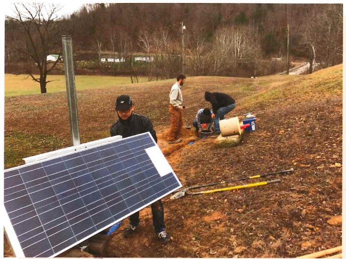
Lifang Zhang, Seth Carpenter, Junjie Sun, and Andrew Holcomb install seismic station EK-36 at Chapman in eastern Kentucky.
