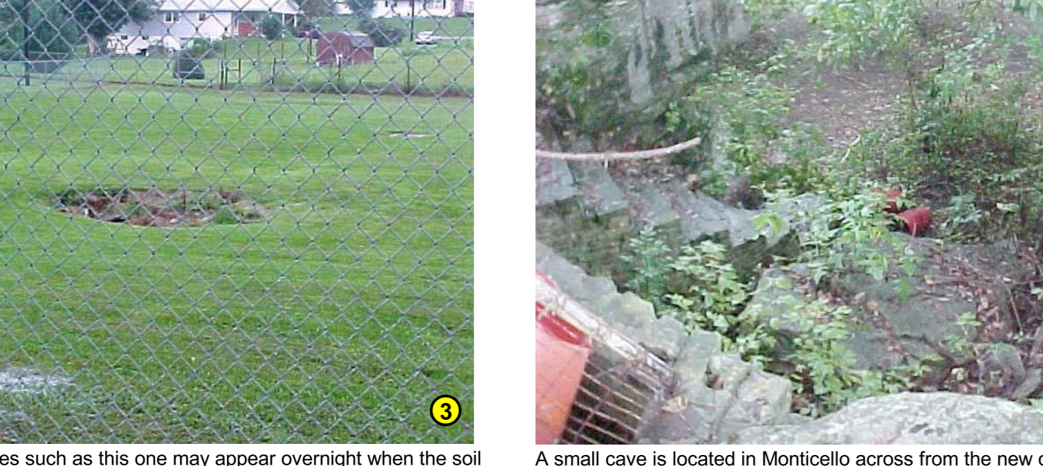
Cover-collapse sinkholes such as this one may appear overnight when the soil plug at their base collapses into a fracture or cave in the underlying limestone. These are direct conduits to the local aquifer, and as such are susceptible to contamination by garbage dumping and accidental spills. They are also hazards to public safety. Photograph by Bart Davidson, Kentucky Geological Survey.
