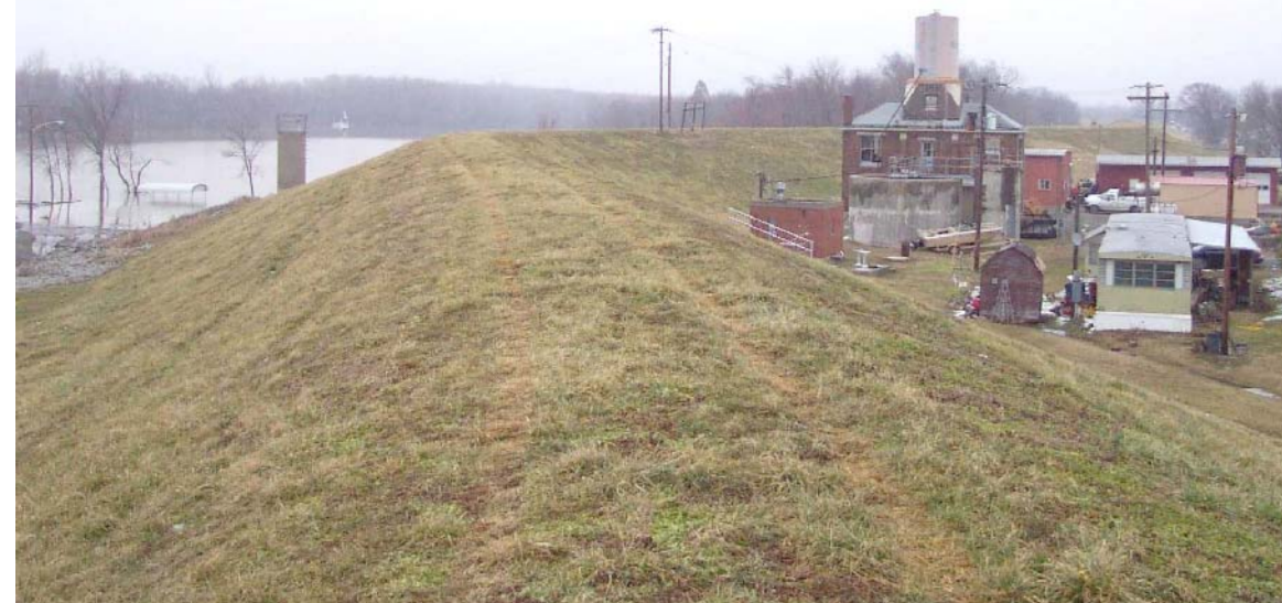
The Uniontown levee was constructed to hold back Ohio River floodwaters. An earthen levee also protects the city of Sturgis. Photo by Glynn Beck, Kentucky Geological Survey.
