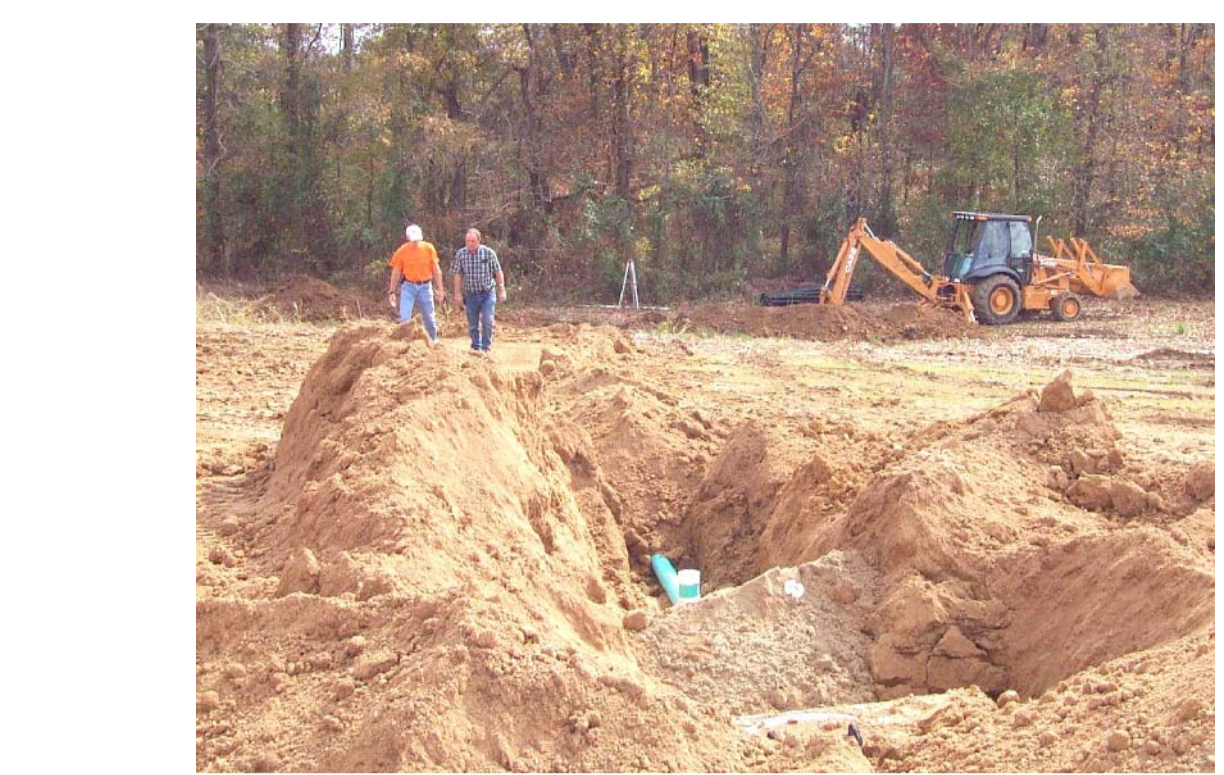
The well-drained soils in Graves County are conducive to the use of septic tanks with lateral lines. The unconsolidated sediment makes for easy excavation. In areas where the soils are not well-drained, unconventional methods to handle waste may be needed. Photo by Glynn Beck, Kentucky Geological Survey.
