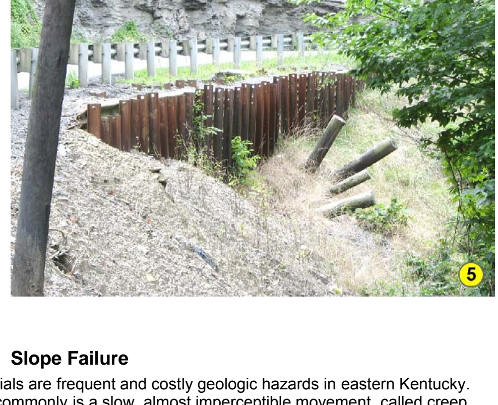
Slope Failure Mass movements or landslides of surficial materials are frequent and costly geologic hazards in eastern Kentucky. The failure of the slope may be rapid, but more commonly is a slow, almost imperceptible movement, called creep, of a few inches per year. Whether rapid or slow, the end results and damage are similar and costly, broken plumbing, cracked walls and foundations, cracked streets and sidewalks, and commonly total loss of the structures. Virtually all units containing shale on slopes are subject to landslides. Gravity is the main driving force, but water nearly always plays a critical role by adding weight and lubricating the particles in the weathered shale. Cutting into or overloading a slope with structures and fill can also be major contributing factors. Precautions include taking care of all surface-water runoff by making certain that all runoff from roofs, gutters, patios, sidewalks, and driveways is carried well away from and toward the house, diverting drainage from areas sloping toward the house; cutting into natural slopes as little as possible and avoiding the use of fill; and trying to place the foundation of the structure on undisturbed bedrock. When in doubt, consult an engineering geologist or a geotechnical engineer. Relict landslides can also be easily reactivated. Look for unusual bulges or cracks in the slope, tilted or curved trees, springs coming out onto the hillslope, and tilted and cracked sidewalks, streets, and retaining walls.
