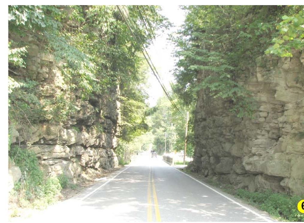
Construction on Shale Hillslope construction can cause earth movements if not properly planned. Photos by Paul Howell, U.S. Department of Agriculture, Natural Resources Conservation Service.
