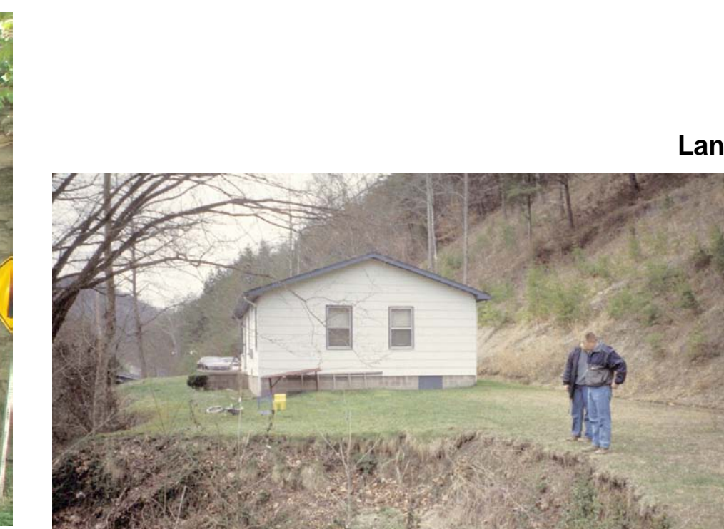
Construction on Shale Hillslope construction can cause earth movements if not properly planned. Photos by Paul Howell, U.S. Department of Agriculture, Natural Resources Conservation Service.
