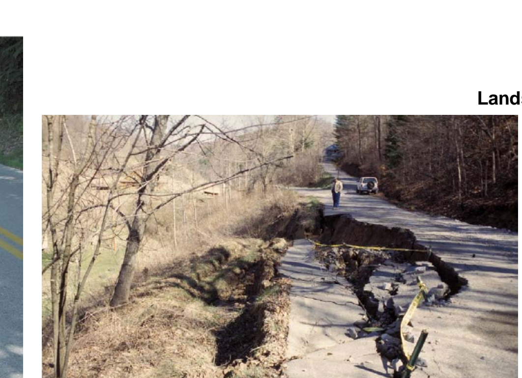
Roadcuts cut into shale often require additional support to reduce pavement failure, as seen in this section along Ky. 708 in unit 3. Photo by Dan Carey, Kentucky Geological Survey.
