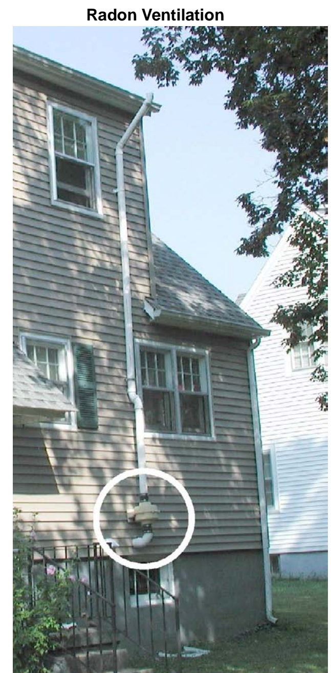
Ventilation system removes radon from the basement area of this home. Photo by Dan Carey, Kentucky Geological Survey.
