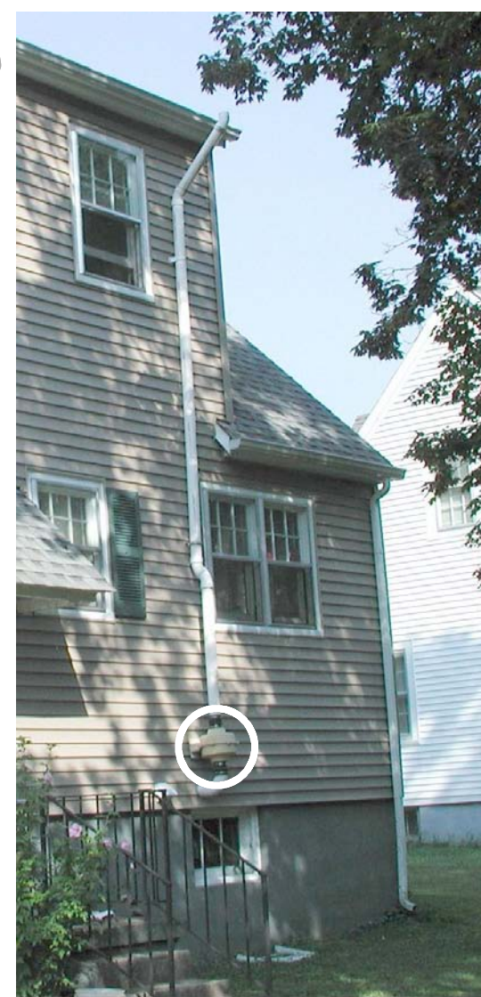
Ventilation system removes radon from the basement area of this home built on black shale. Photo by Dan Carey, Kentucky Geological Survey.
