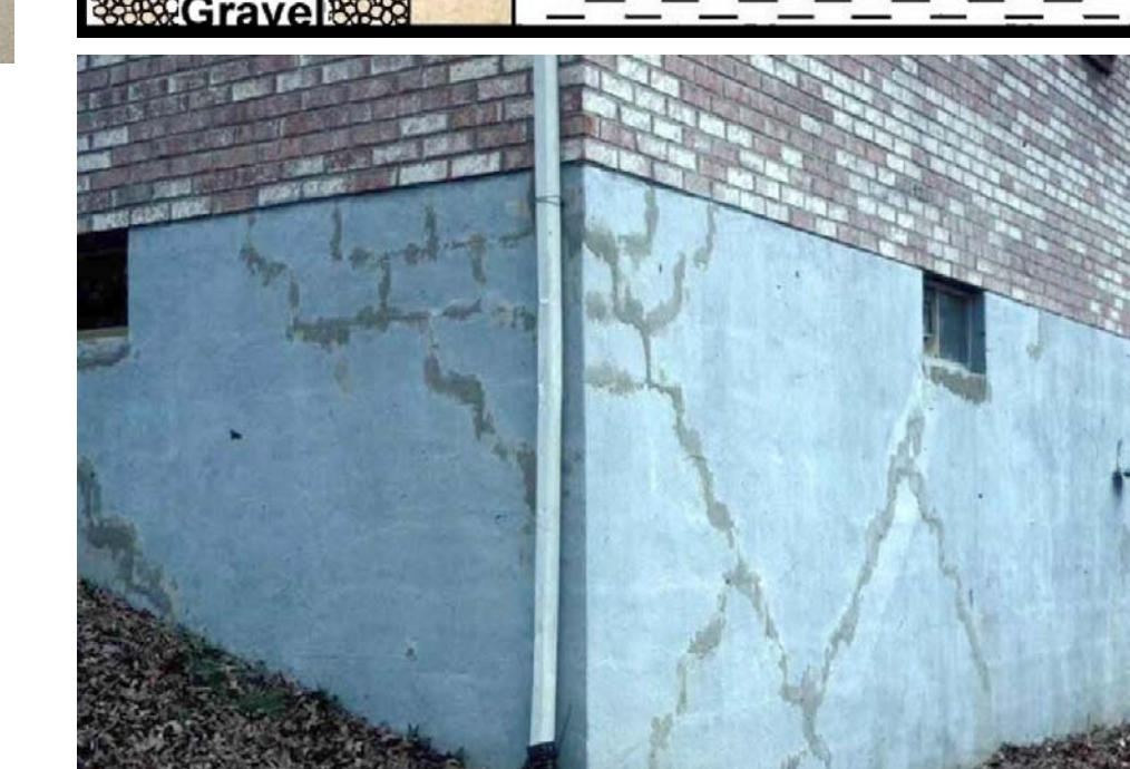
Some shales and the soils derived from them swell when exposed to water or air. These swelling shales and soils can have severe impacts on building foundations and other structures (e.g., bridges, dams, roads). Photo by John Kiefer, Kentucky Geological Survey.
