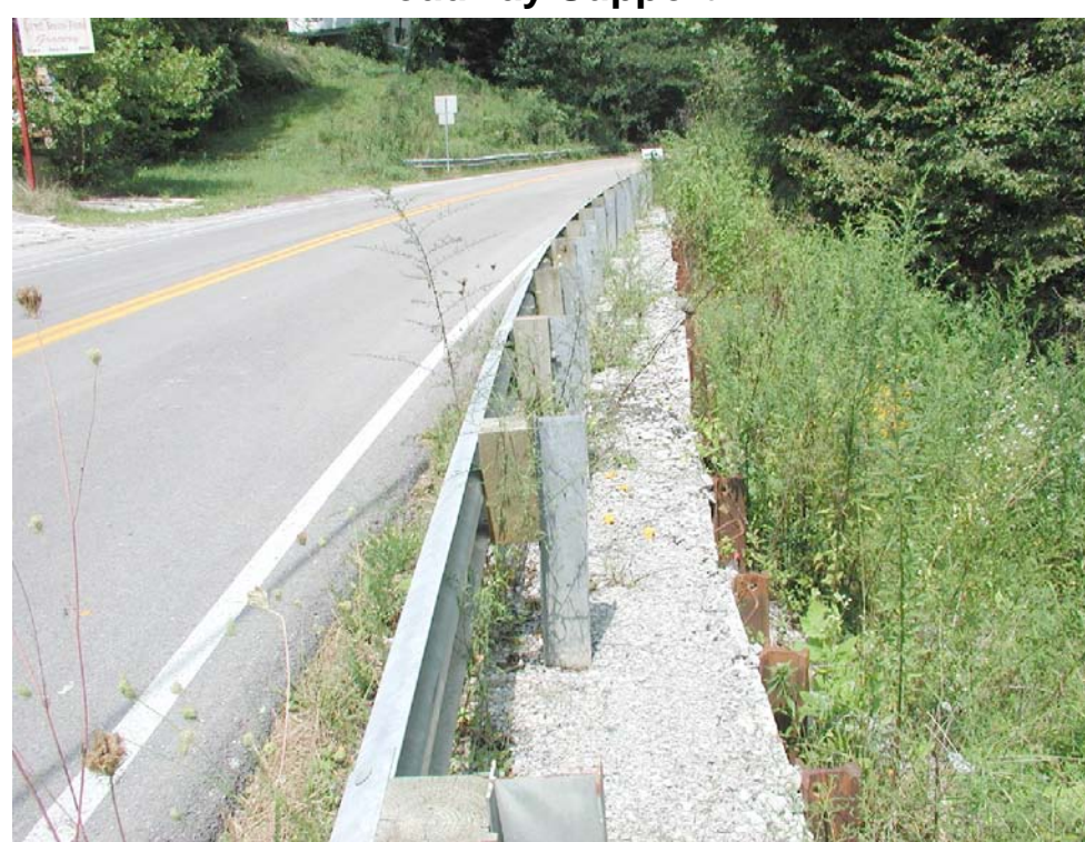
Drainage management and roadway support are mandatory in steep slope areas that are common in McCreary County, particularly if shale units are encountered. Photo by Randy Paylor, Kentucky Geological Survey.
