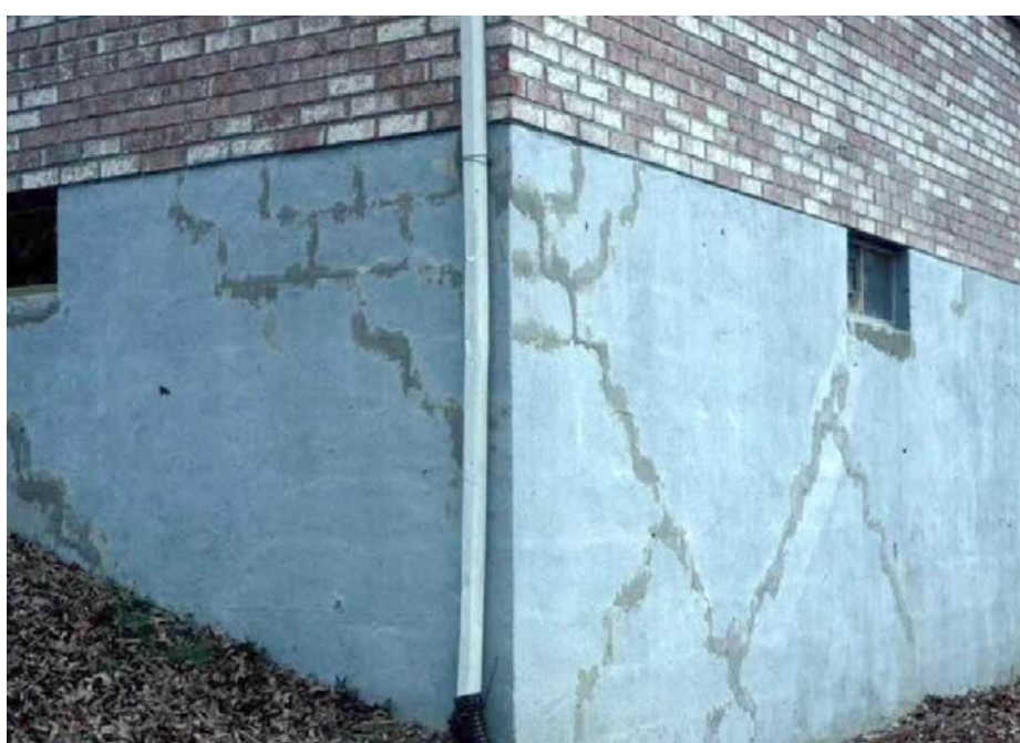
Some shales, and the soils derived from them, swell when exposed to water or air. These swelling shales and soils can have severe impacts on building foundations and other structures (e.g., bridges, dams, roads). Photo by John Kiefer, Kentucky Geological Survey.
