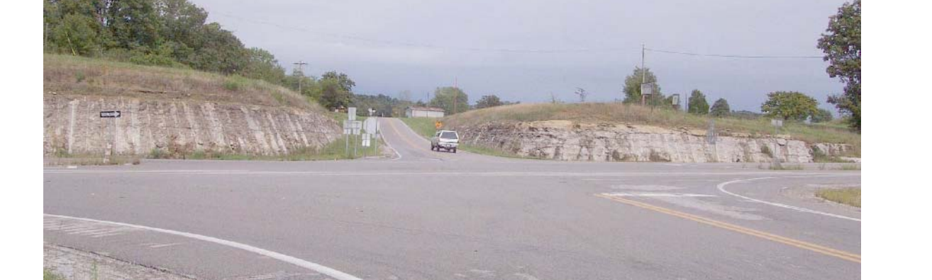
Because of thin soil cover and hilly topography in certain areas of the county, rock excavation is required during road and other types of construction. Photo by Glynn Beck, Kentucky Geological Survey.
