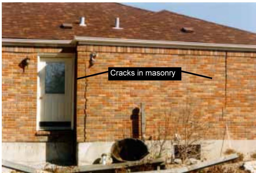
A cover-collapse sinkhole caused more than $40,000 in damage to this home near Louisville. Photograph by J.C. Currens.
