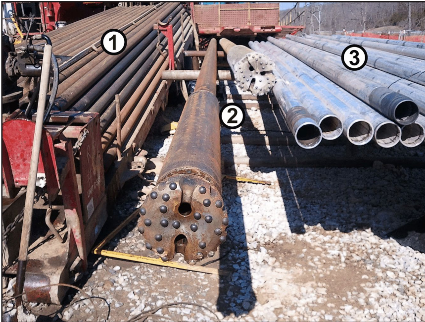
Figure 15. Drilling tools and tubular materials on racks beside the drilling rig, where they were easily accessible to the rig crews during drilling. (1) Drill pipe. (2) Hammer-drill heads. (3) Aluminum core sleeves.
