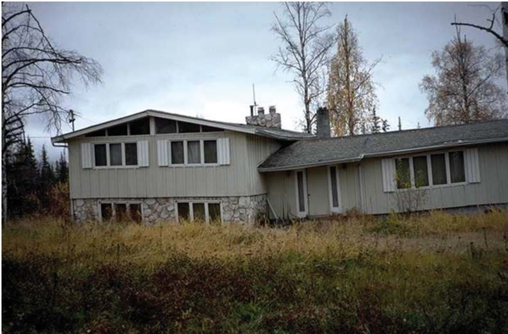
The result of building a conventional foundation on permafrost-affected soils containing massive ice. Heat transfer from the house resulted in melting of the ice and displacement of the foundation. (Photo by Alaska NRCS staff.)
