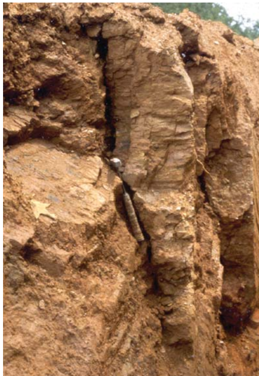
Fissures developed in a trench wall along natural zones of weakness in the soil profile. Note hand pick for scale.
