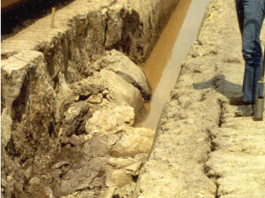
Tension cracks forming parallel to a trench excavation.
