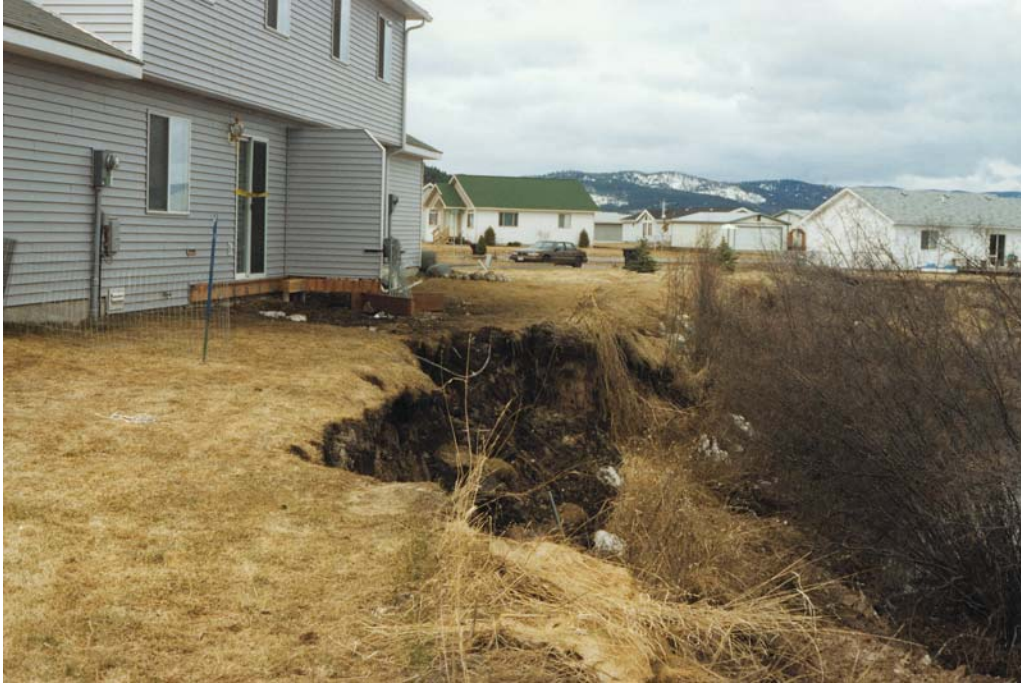
Landslides are hazardous. (Photo by Chuck Gordon, USDA, NRCS.)
