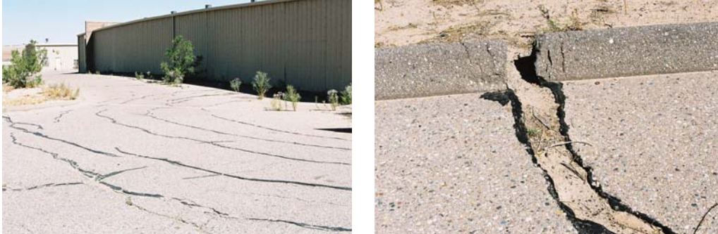
Concentric cracks caused by soil collapse near abandoned buildings in New Mexico. (NRCS photos.)
