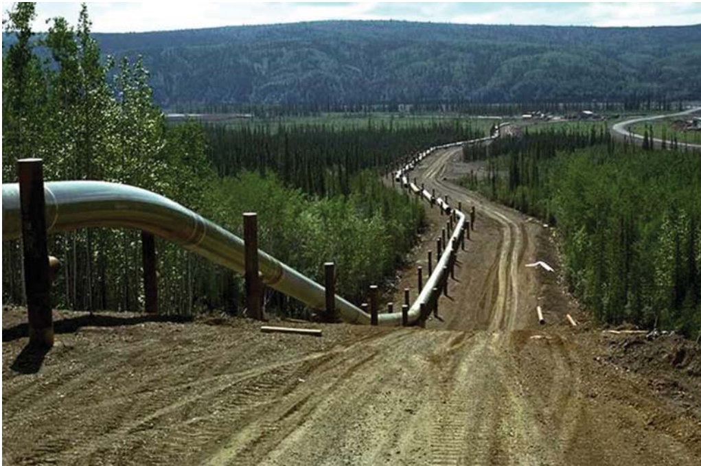
Permafrost-affected soils with loamy textures become saturated and unstable if allowed to thaw. In areas of these soils, the trans-Alaska oil pipeline is elevated above the ground. (Photo by Alaska NRCS staff.)
