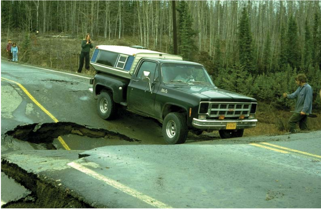
Collapse of a section of the Alaska Highway in 1982 after massive ice under the roadbed melted. (Photo by Joe Moore, USDA, NRCS).
