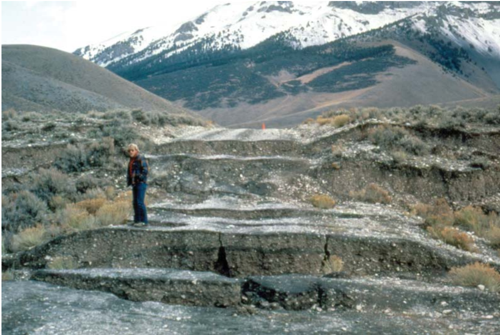
Severe road damage caused by an earthquake in east-central Idaho. (Photo by Karl Hipple, USDA, NRCS.)
