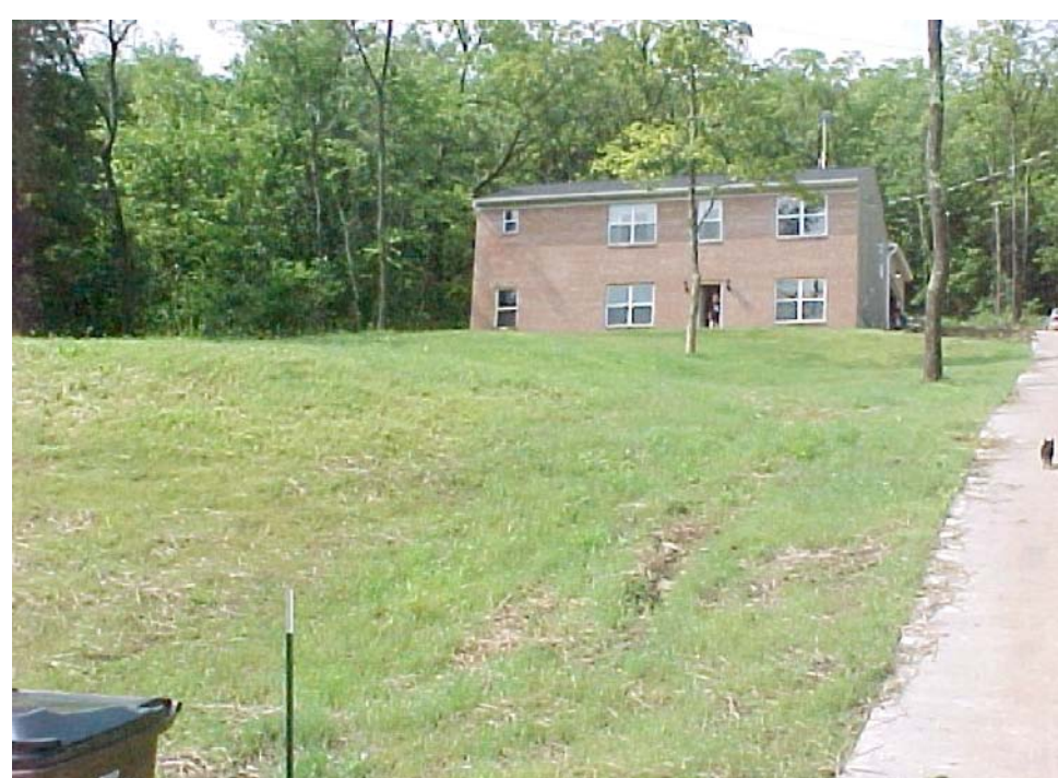
Home built on unit 2 showing initial signs of slope failure--cracks in concrete, leaking basement, and slumping septic system installed on downslope front yard. Photo by Warren Anderson, Kentucky Geological Survey.
