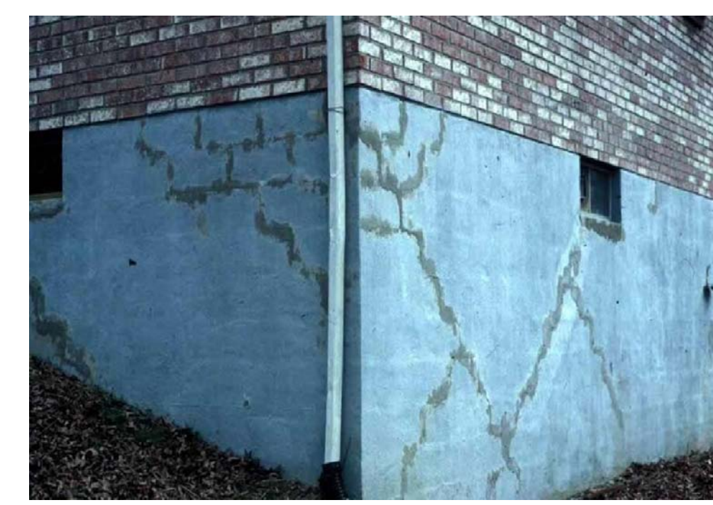
Some shales, and the soils derived from them, swell when exposed to water or air. These swelling shales and soils can have severe impacts on building foundations and other structures (e.g., bridges, dams, roads). Photo by John Kiefer, Kentucky Geological Survey.
