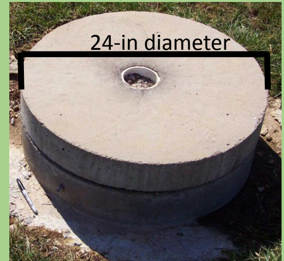
Bored well (Cement tile casing)
